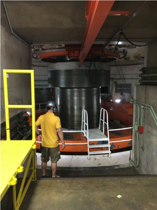
Figure 6.32. Spinning turbine, inside the generation unit.
